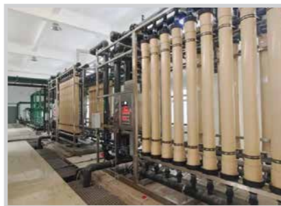
Qinghai Kunlun Gold Refinery – Reclaimed Water Reuse Project
