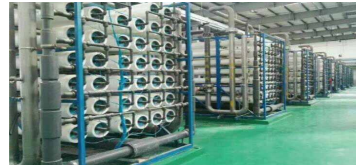
Koubei Water Plant, Chaoyang, Liaoning
