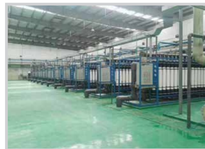
Ningdong Base – Nanhu Reclaimed Water Treatment
