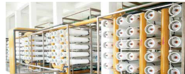
Xilinhot Municipal Water Plant
