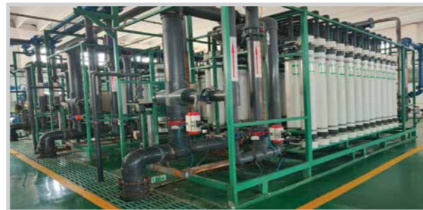
Yanggu Senquan Water Plant Co., Ltd. – Wetland Reclaimed Water Reuse Project
