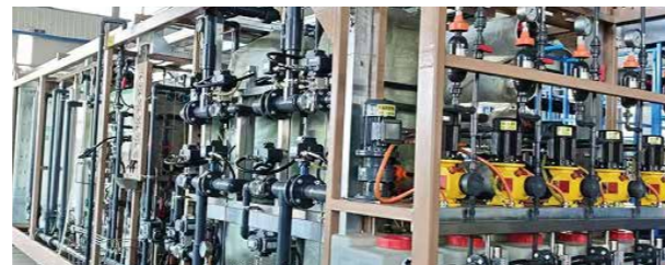
Wuxi Longi Hydrogen Energy Technology Co., Ltd.
