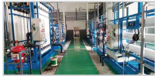
Miyun District Urban Management Committee, Beijing (Reclaimed and Wastewater Treatment Project)
