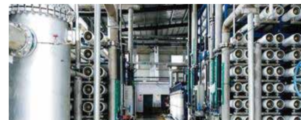
Woniushan Water Plant, Yantai, Shandong
