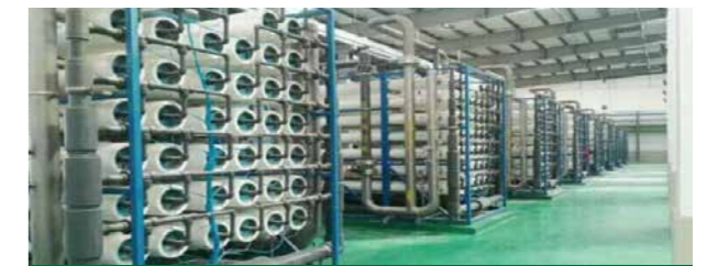
Rongcheng City Natural Gas Cogeneration Project
